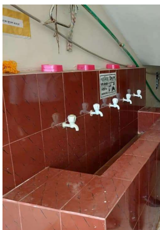
Fig. 9 water collection basin of 5 outlet
